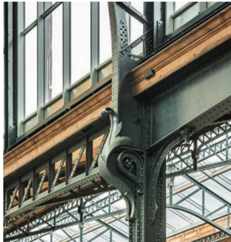
Top centre: The timber pavilions had to be designed so they could be assembled by small plant in the existing structure
