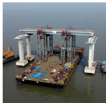
The client for the Mumbai Trans Harbour Bridge (above) is reportedly considering adding Metro lines later
